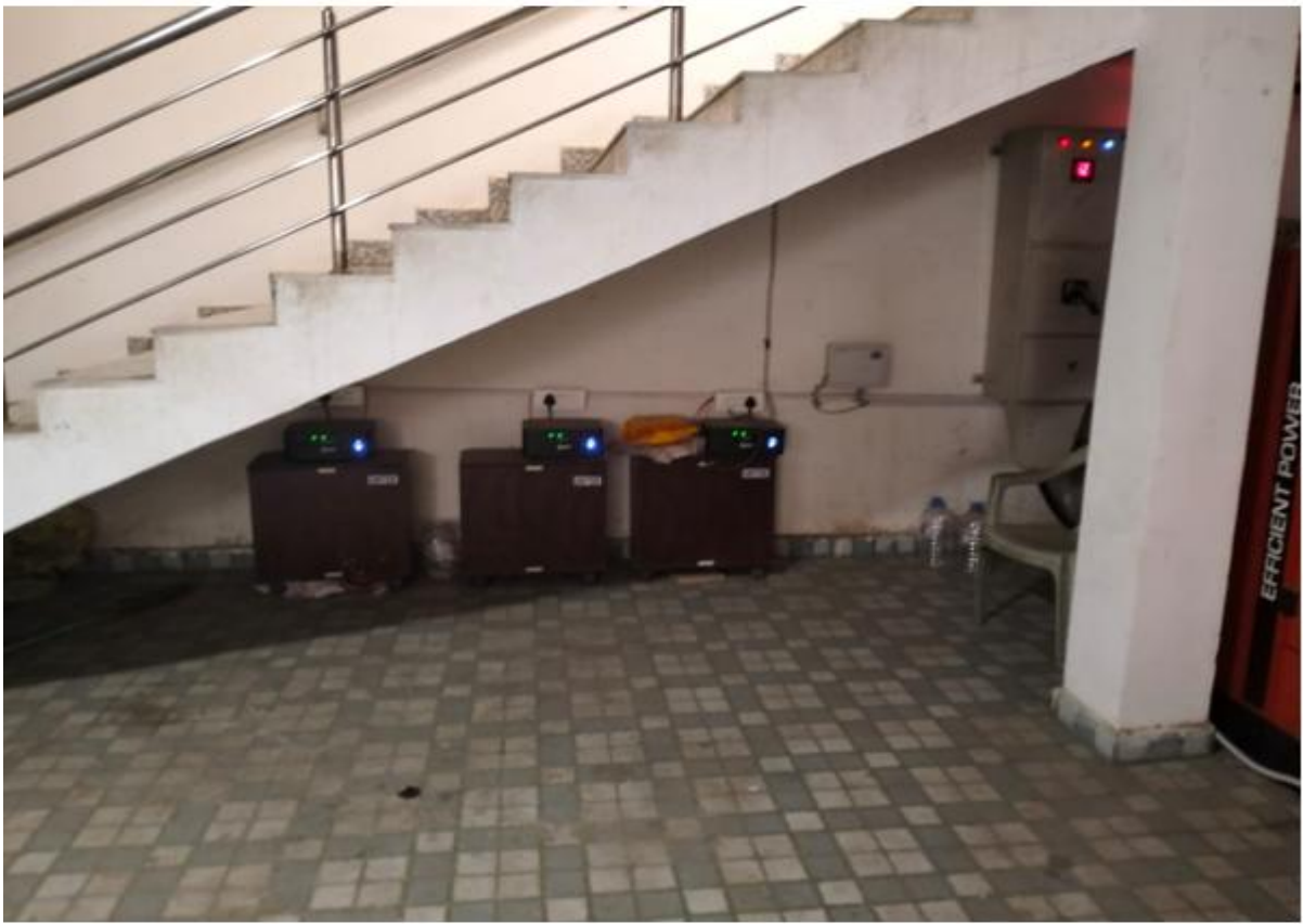
Pic 4: The source of electricity generators and generator in the new building.
