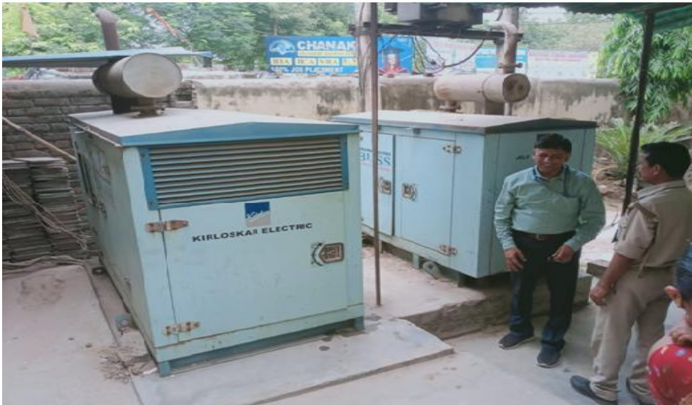
Pic 3: The source of electricity such generators and transformer in old building of the college.
